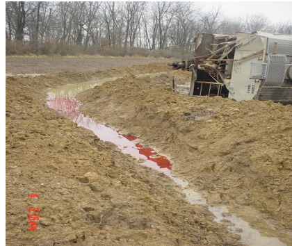
Interceptor trench train derailment
