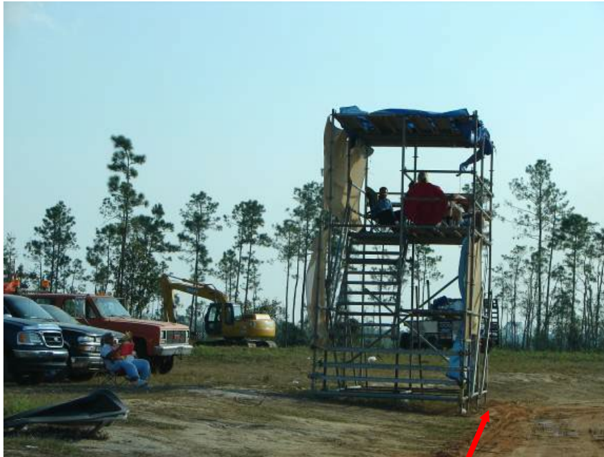
No Cone or Barrier between traffic and QA Tower
