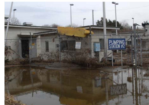
Aftermath of Japan earthquake 2011: potential grey/black water
